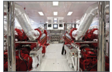
Marine Engine Rooms
