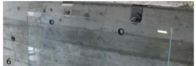
6 Insert the Chloroprene grommets into the holes in the glass panels, then align over the fittings.
